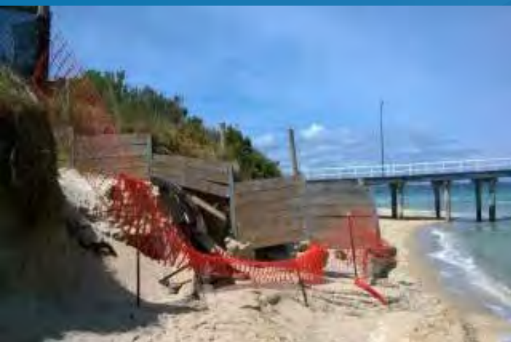
Impacts on infrastructure
