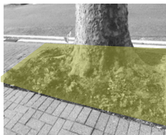
Undesirable weed growth surrounding tree base due to lack of pit infill cover.
