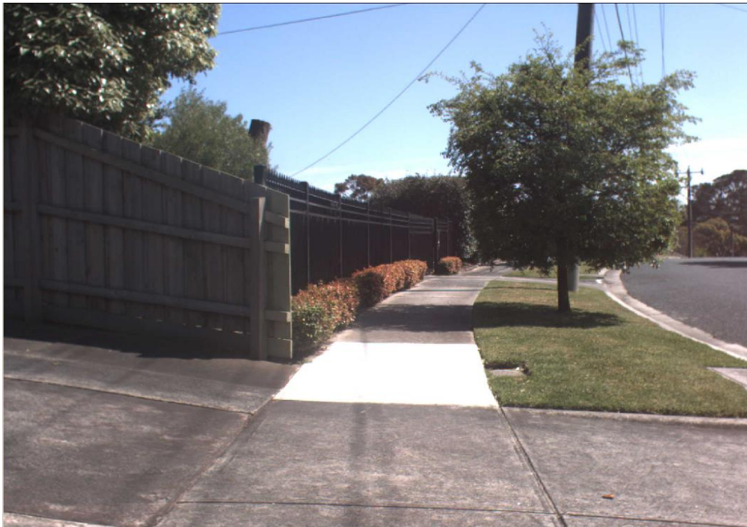
Footpath 35540,1,3 – Bangor Drive, Frankston – Segment 42 years old, assessed as condition 2
