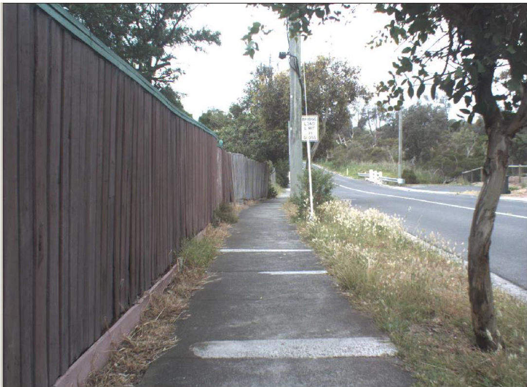
Footpath 11090,1,1 – Armstrongs Road, Seaford – Segment 42 years old, assessed as condition 2
