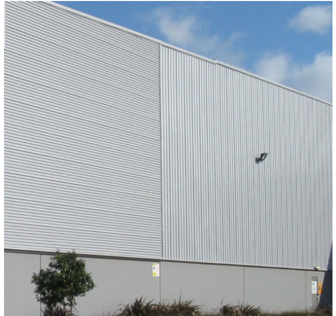
Providing textured panelling and changing the orientation of the panelling can provide for effective articulation
