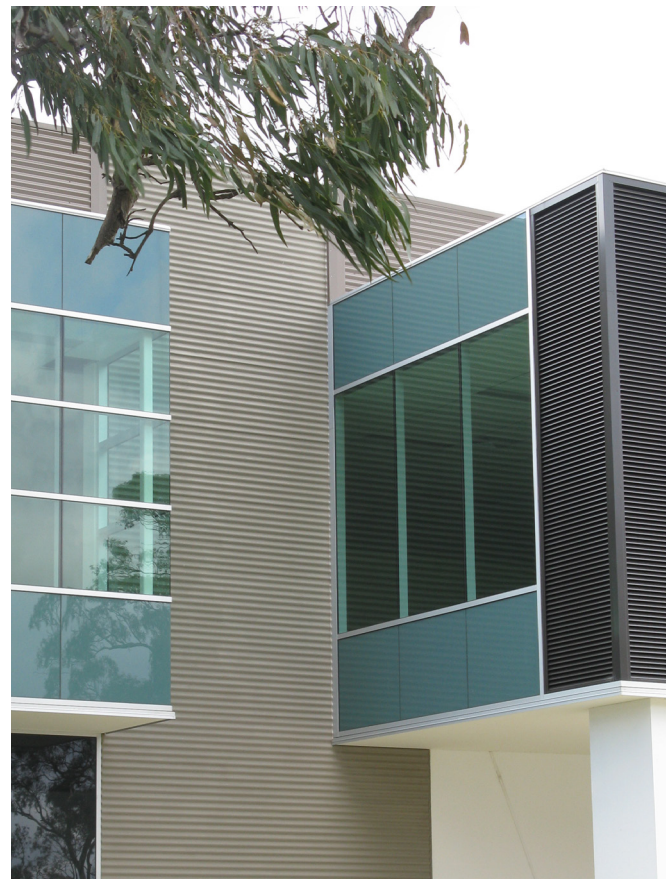
This facade utilises a variety of colours, textures and projected elements to provide effective articulation
