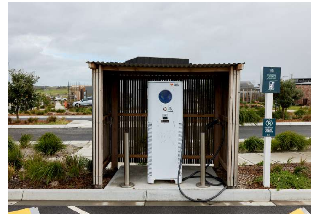
Electric vehicle charging station at The Cape development. Photography by Kim Landy
