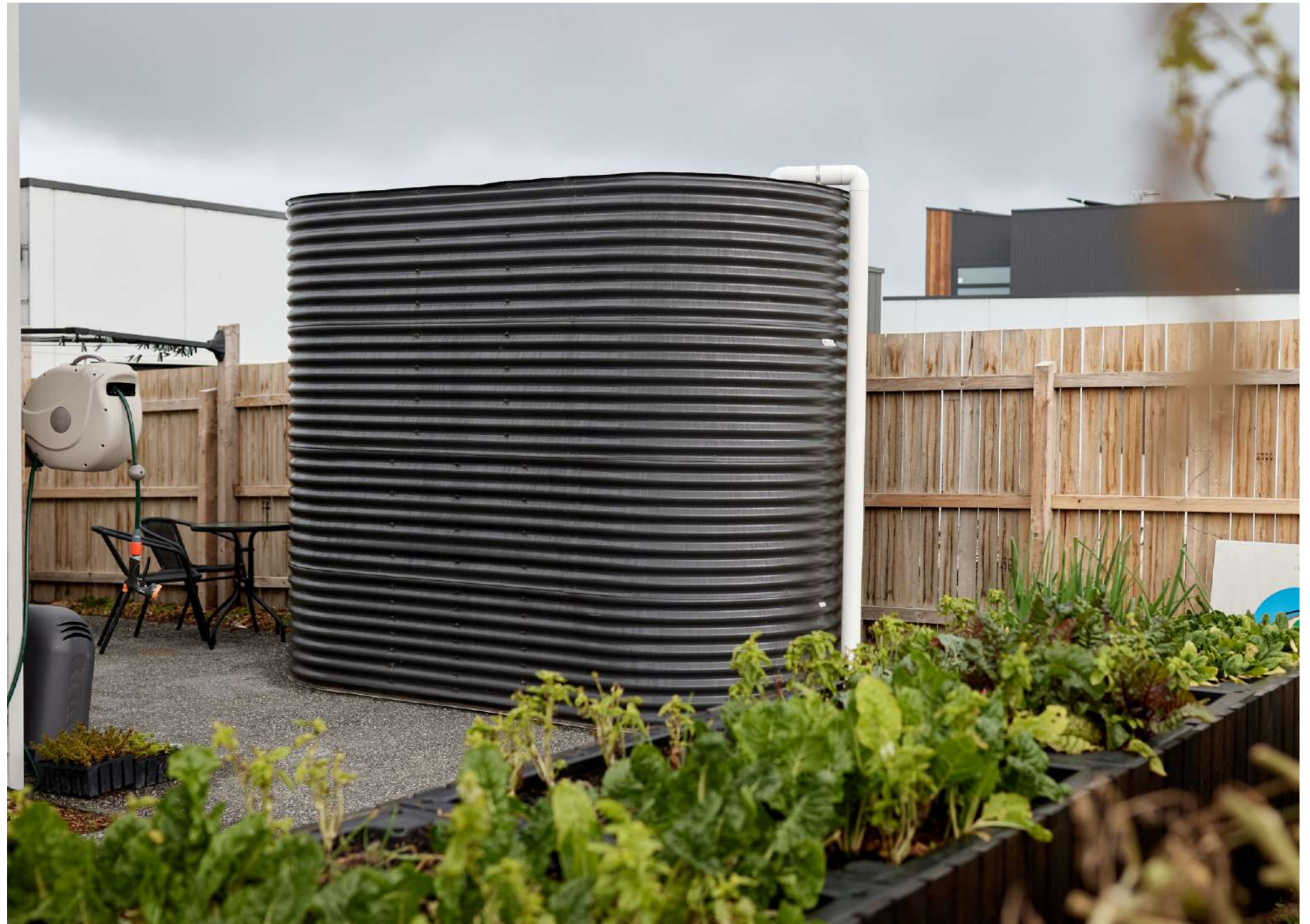
Rainwater tank in rear garden of dwelling at The Cape development. Photography by Kim Landy
