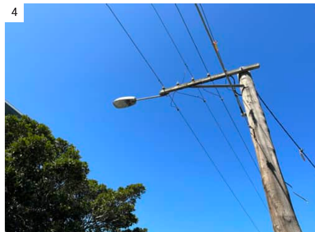
4 Nepean Hwy footpath located poles It was observed a number of legacy street lights were fixed to timber power poles. The S250 light heads are high-pressure sodium lamp types which have a distinctive amber colour temperature. Power poles and exposed cables were observed within this location.
