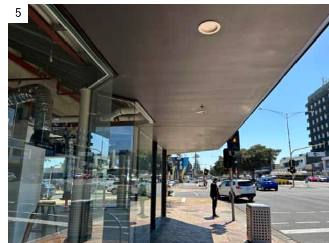
5 Nepean Hwy CBD canopies with lighting Lighting is provided inconsistently by tenants under selected canopies, while other canopies do not have any lighting. In many cases, the canopies baffle the light from nearby roadway light poles resulting in an inconsistent light level for users as they walk along the footpath.
