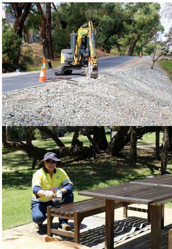
Photo: 2 Works being completed at Valley Road, Langwarrin and maintenance works in progress at George Pentland Botanic Gardens.
