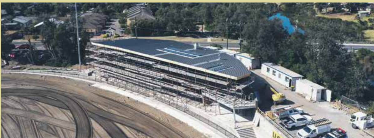
Amazing progress at the RF Miles construction site in Seaford, as the $9.147 million redevelopment, funded by Council, Victorian and Federal Governments, takes shape.
