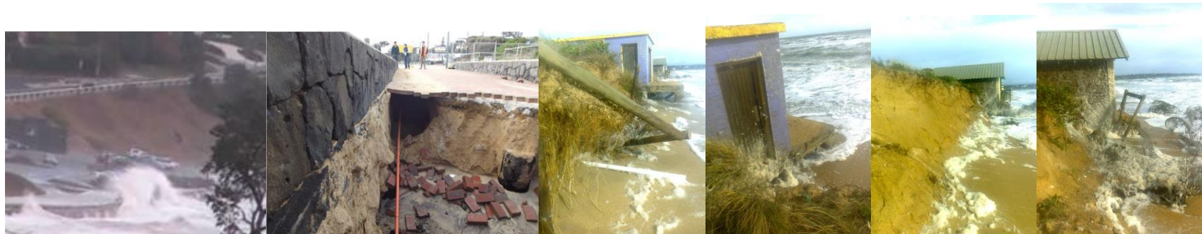
Figure 34: Storm damage and erosion of foreshore infrastructure and beaches at Frankston foreshore
