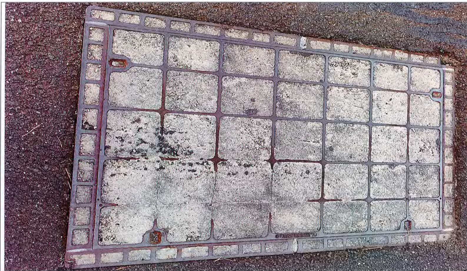
Ductile Iron and concrete access cover (heavy vehicle traffic)
