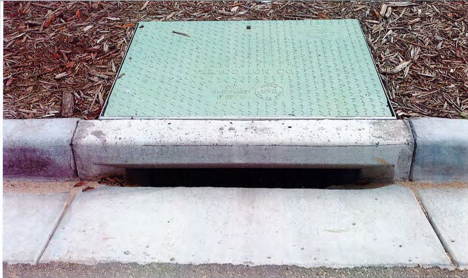
Concrete lintel & polymeric cover
